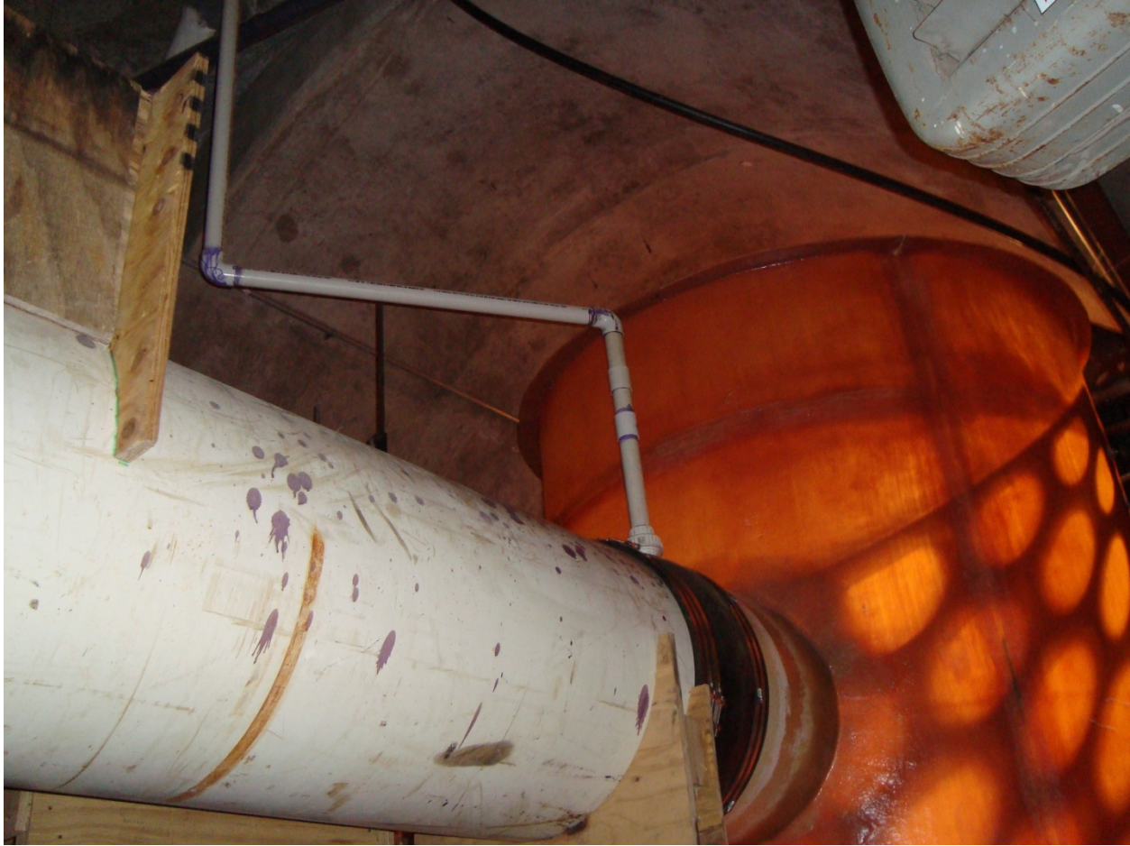
Figure 2-7: A view of the slurry pipe used to feed sediment into the sump.
